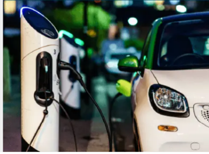
EV charging station
