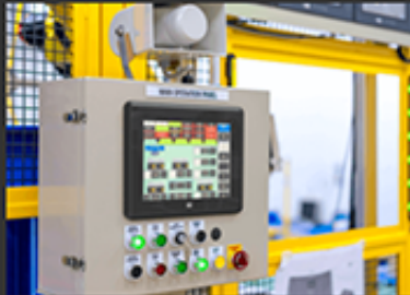
Process Automation System
